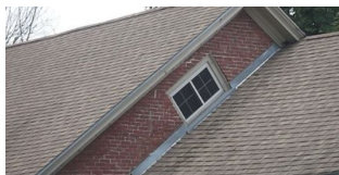
A very unusual example of a diagonal window set in a brick wall
