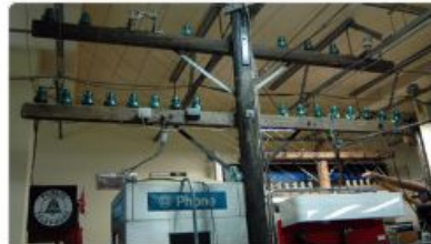
The Outside Plant
